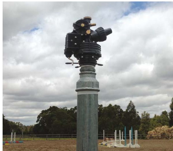
Turbina ST-1600-HS-BR instalada
